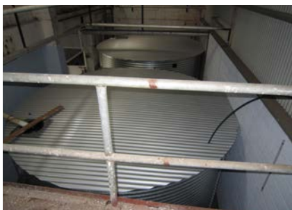
Boiler house rainwater storage tanks 34,400 each.
