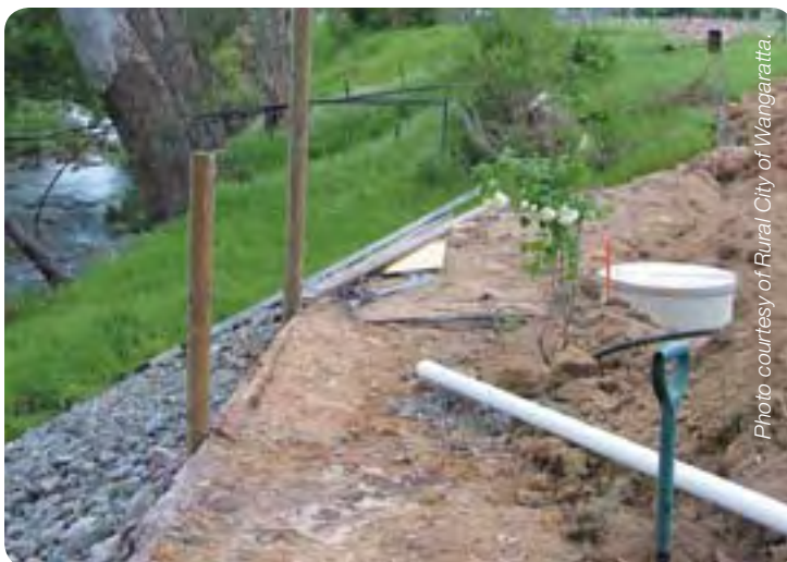
Unacceptable septic tank installation located too close to a waterway.
