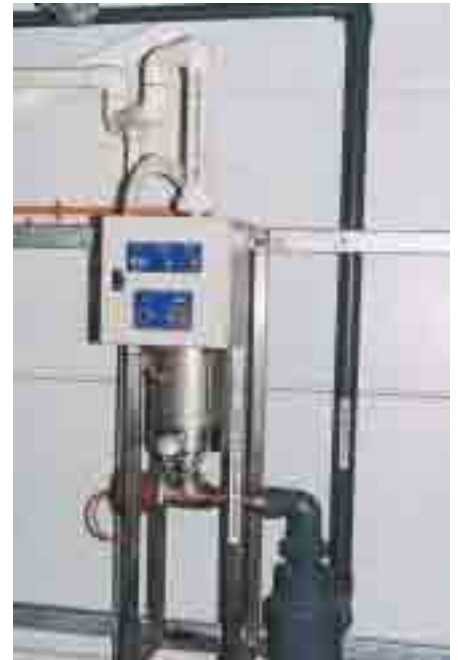
Figure 12 Ozone off-gas destructor
