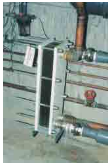
Figure 39 Gas fired direct pool water heater
