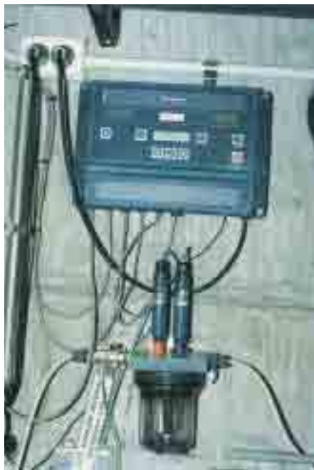
Figure 19 Chemical sensors installed in a side-stream loop
