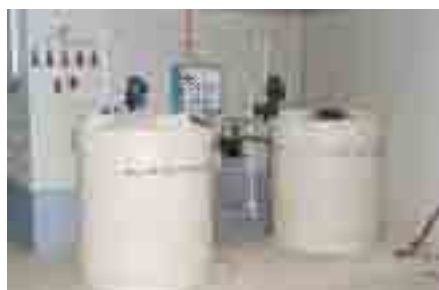
Figure 35 Dosing tanks with mixers for adding coagulant
