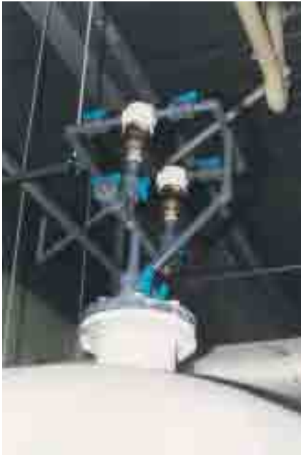
Figure 33 Filter off-gas bleed and collectors
