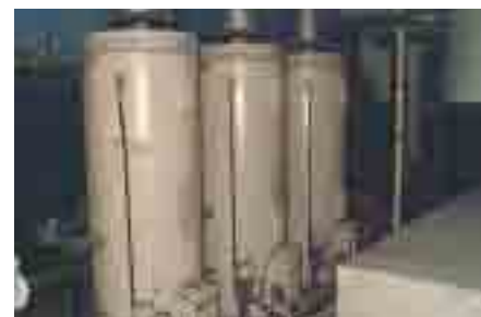
Heavy duty or electric boilers supply water to heat exchanger closed loop.
