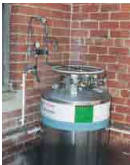
Figure 13 Carbon dioxide tank
