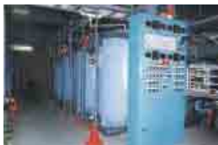
Figure 30 plant room with multiple filters
