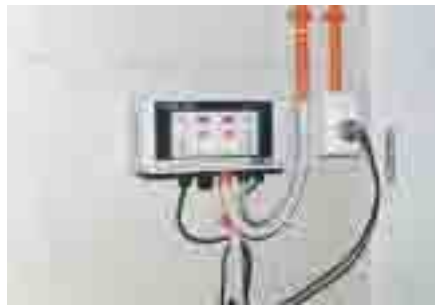
Figure 11 Ozone leak detector
