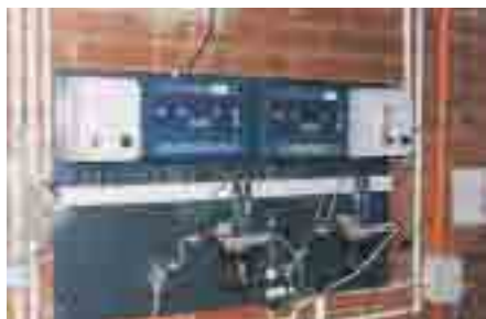
Figure 18 Pool control panel and chemical measuring station
