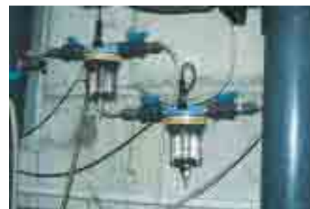
Figure 9 Pool water treatment with ozone and hypochlorite
