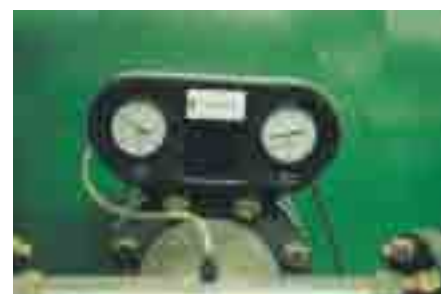
Figure 36 Pressure differential gauges
