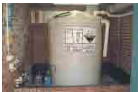
Figure 7 Bulk sodium hypochlorite container in bund
