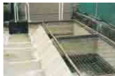
Figure 32 Old style gravity sand filter beds and backwash channel
