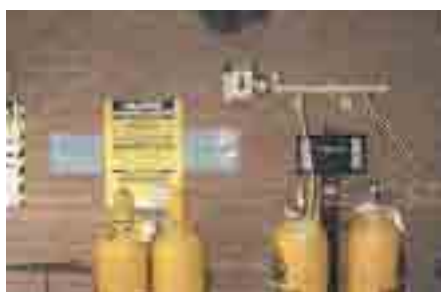
Figure 6 Chlorine gas, weight scales and regulator
