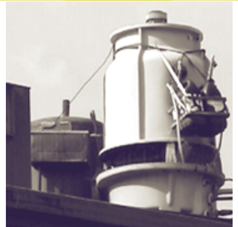
An example of a cooling tower
