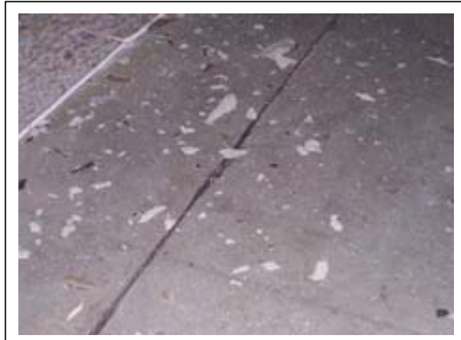
Figure 15 Spalled pieces of A/C sheeting on floor, away from Test Rig
