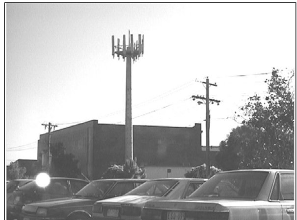
Figure 4. Cellular mobile phone base station.
