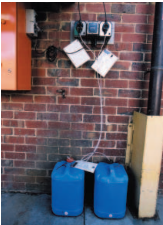
Automated biocide dosing: This device has a timer which controls a pump to inject a pre-set volume of biocide into the water
