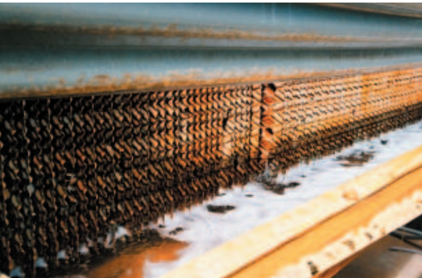
Cooling tower with basin exposed to sunlight: This cooling tower does not have sunlight protection to the side and basin of the tower
